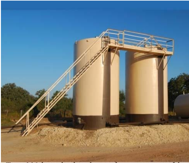
Twin 210 barrel oil tanks inside containment dike
